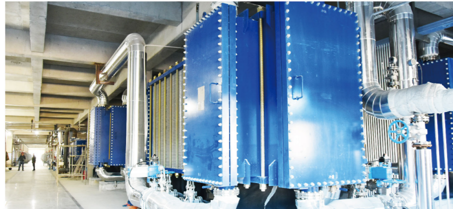
液糖化车间-换热器 Liquid saccharification workshop - heat exchanger
